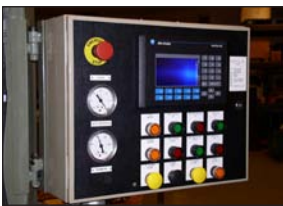
Multiple Level Control Packages
